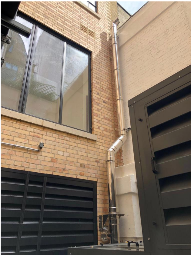
Generator exhaust flue
