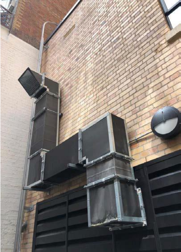
Smoke extract duct
